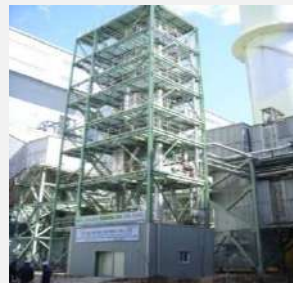
0.5MW CCS plant
