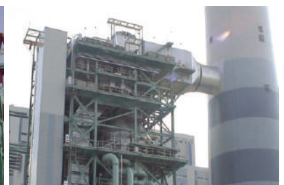
• Hadong Thermal Power Plant
