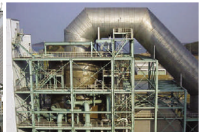
• Dangjin Thermal Power Plant
