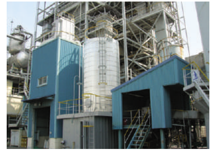
• CFBC Boiler, LG Chem
