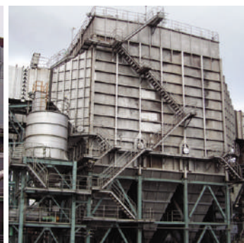
• Kasima Power Plant
