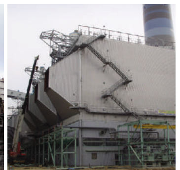
• Taean Thermal Power Plant Units 7~ 8
